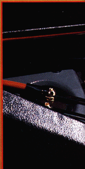
RIGHT - The system's second battery has half farad capacitors on either side connected with hand made Busbars constructed by owner Randy Wilbur.
